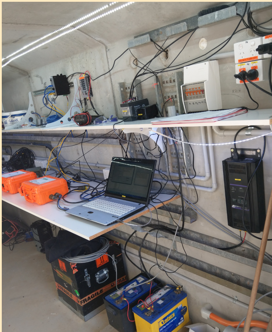
Two not so new batteries and a recycled battery charger.
