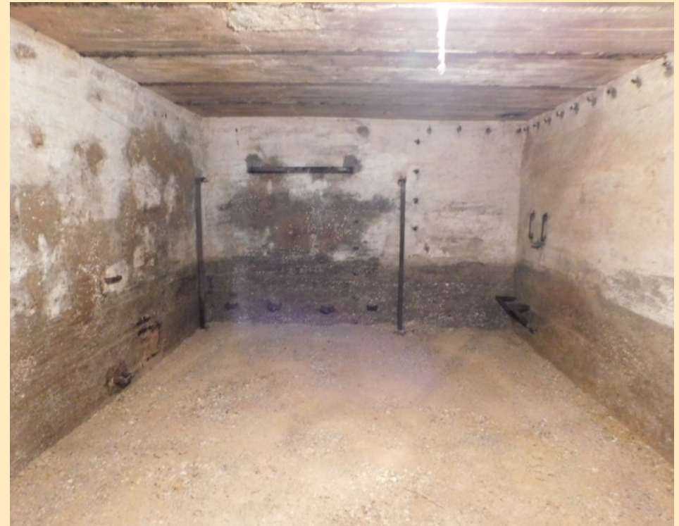
Figure 11: The instrument chamber hosting a seismometer and a tilt meter
