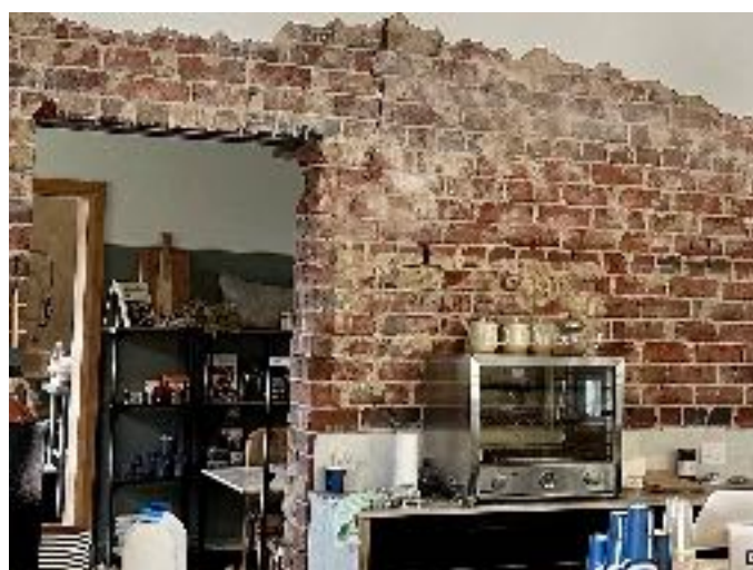
Photo One might classify this wall as vulnerable masonry at a business in Boorowa NSW, about 20k SE of the epicentre where the horizontal pga may well have exceeded 0.1g briefly
